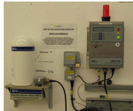
Fig 4: Installed Radiation monitor.
