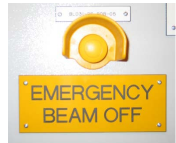
Fig 5 Emergency Beam off button.
