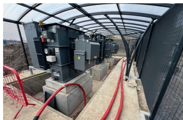
Figure 4: The high voltage substation
