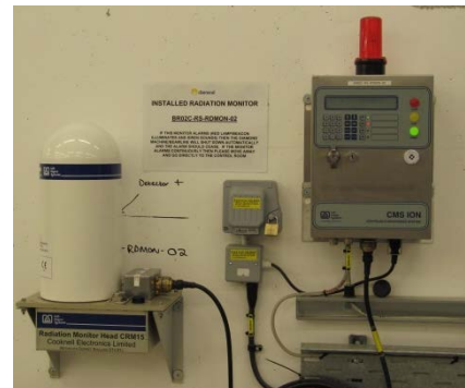
Fig 4: Installed Radiation monitor.
