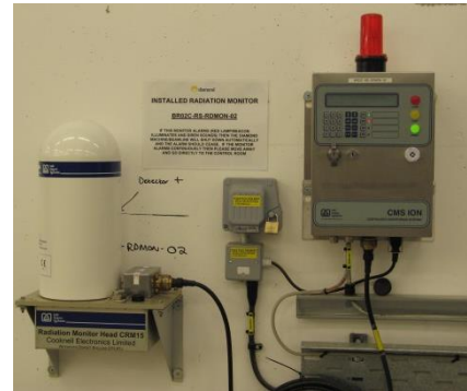
Fig 5 Installed Radiation monitor
