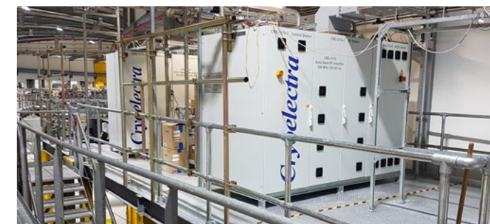
Two new 120 kW solid-state 500 MHz amplifiers installed on a new platform in readiness for Diamond-II.
