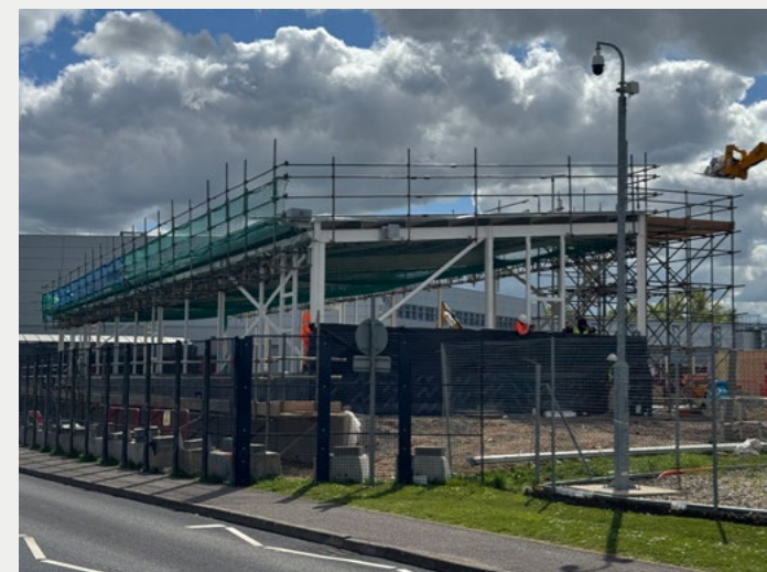
1MW Data Centre
