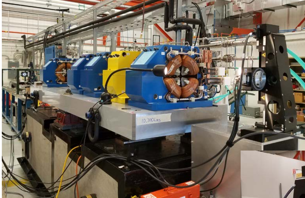
Upstream and outboard end of DMM assembly
