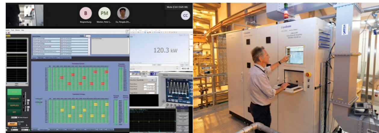
Figure 2. left - 120 kW solid state amplifier Site Acceptance Test witnessed via video link, right - amplifier installed at Diamond.
